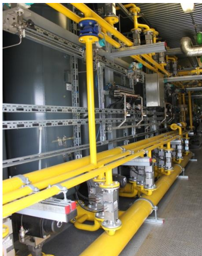
Figure 66: Pressure Swing Absorption (PSA) technology at Aiterhofen, Germany (Source: Rutz)
