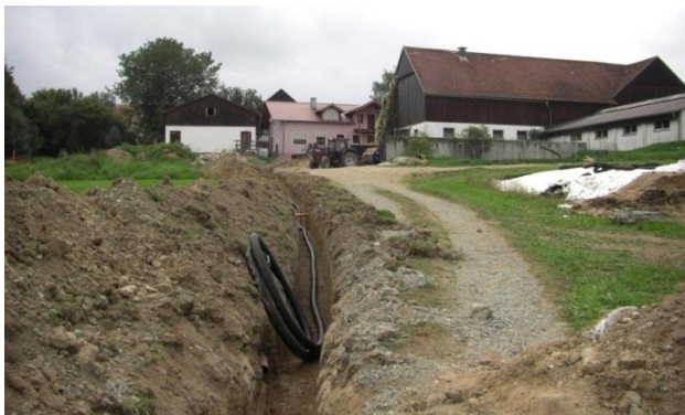
Figure 12: Installation of a heat pipe to the buildings of a farm (Source: Thermaflex Isolierprodukte GmbH)
