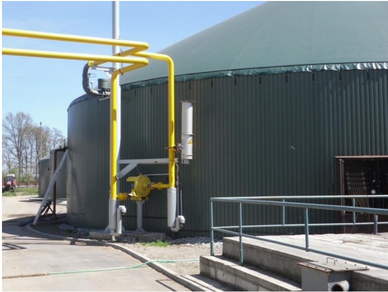
Figure 63: Start of biogas pipes to a satellite CHP unit to the town of Trebon, Czech Republic (Source: Rutz)
