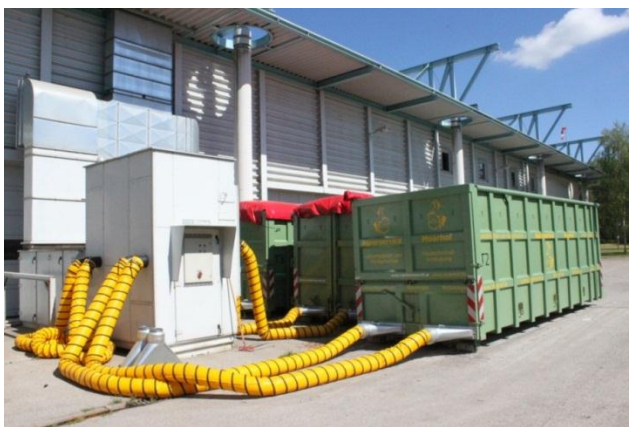
Figure 46: Container and air heating pipes for wood chip drying at a biogas plant in Munich, Germany (Source: Rutz)
