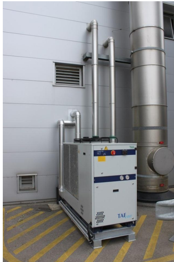
Figure 53: Air-cooled chiller using waste heat of an incineration plant in Austria (Source: Rutz)
