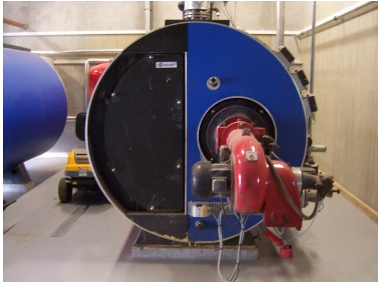
Figure 21: Biogas boiler of 1,500 kW capacity in Denmark (Source: Rutz)
