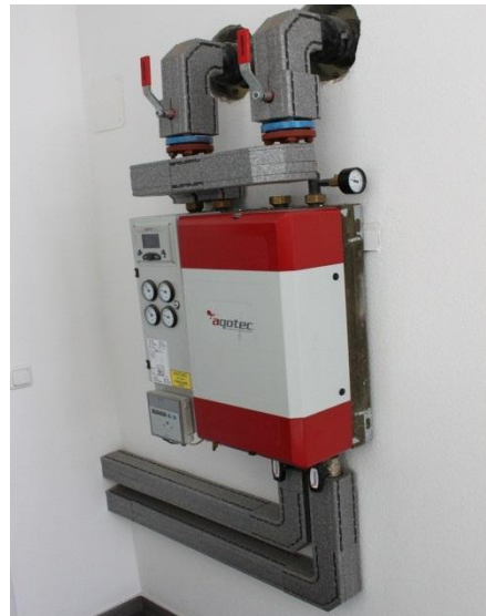
Figure 15: Connection equipment (including a heat exchanger) of an end consumer in Achenal, Germany (Source: Rutz)
