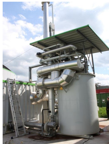
Figure 4: Low calorific value (LCV) burner of a biogas upgrading plant for digester heating in Aiterhofen, Germany (Source: Rutz)
