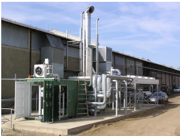
Figure 56: ORC system (using R245fa) of a biogas plant in Dublovice, Czech Republic (Source: GE Energy)
