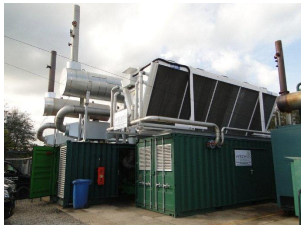
Figure 57: ORC system (using R245fa) (container in the front) and biogas engines (container in the back) of a landfill site in Warrington, U.K. (Source: Verdesis Services UK Limited)
